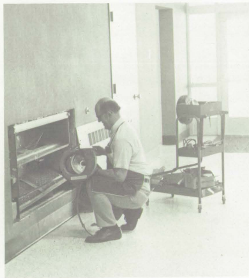
left: Repairing heaters is just one of the duties of maintenance manager Max Ayres.
